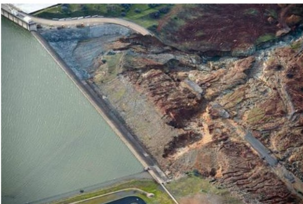
The emergency spillway at Lake Oroville shows signs of damage from the water that spilled over on Feb. 13 in Oroville. Randy Pench - rpench@sacbee.com
